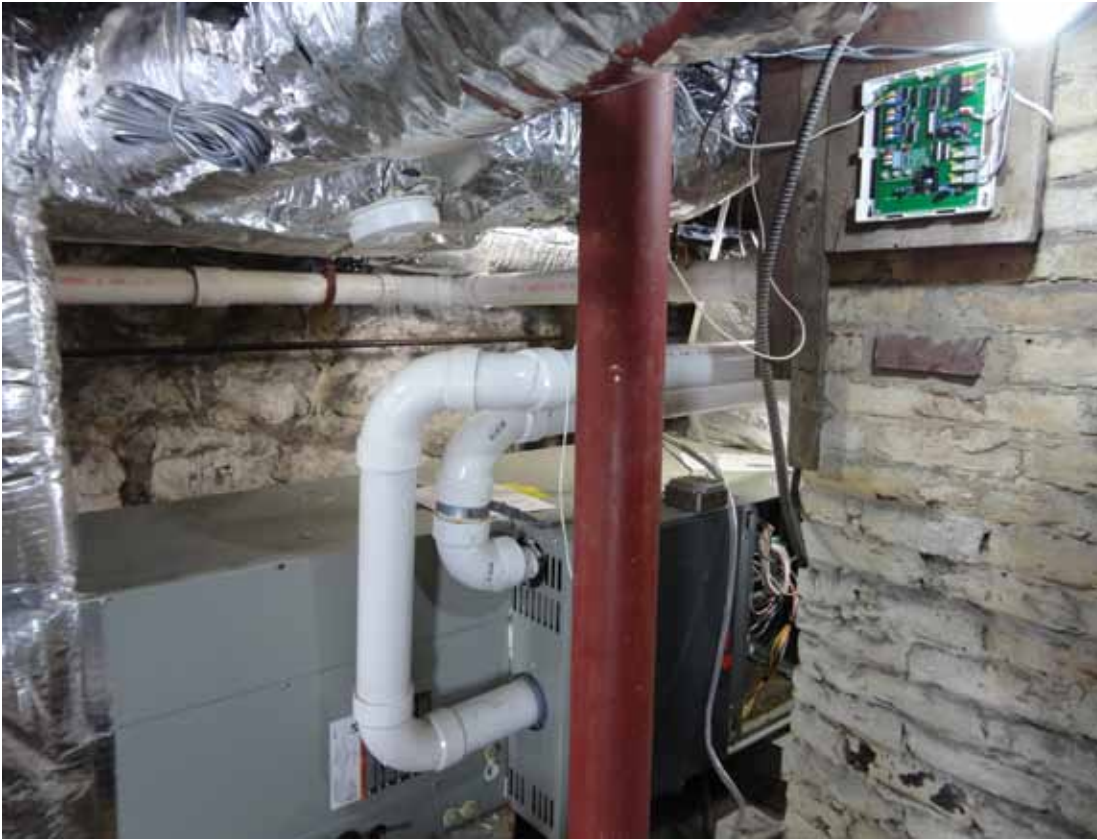
« A three-zone control panel being wired to add zoning to existing system, mounted next to furnace.
